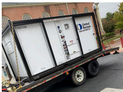
External HVAC unit being used for the cafeteria. By Bryant King
