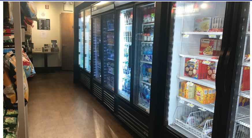
Inside the POD
