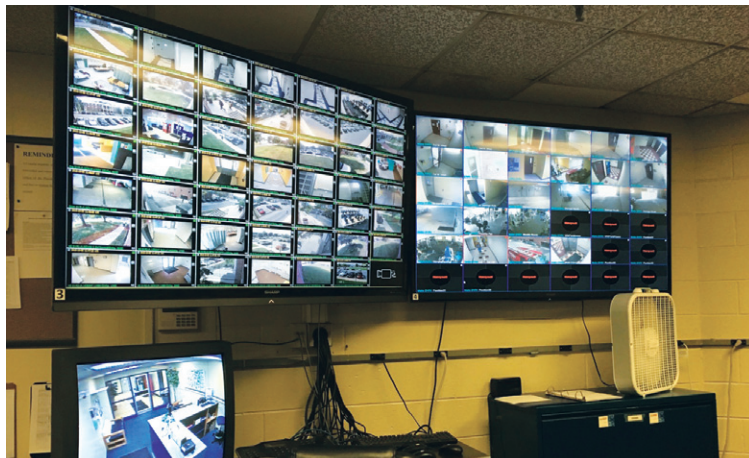
Security camera monitors in the security office
